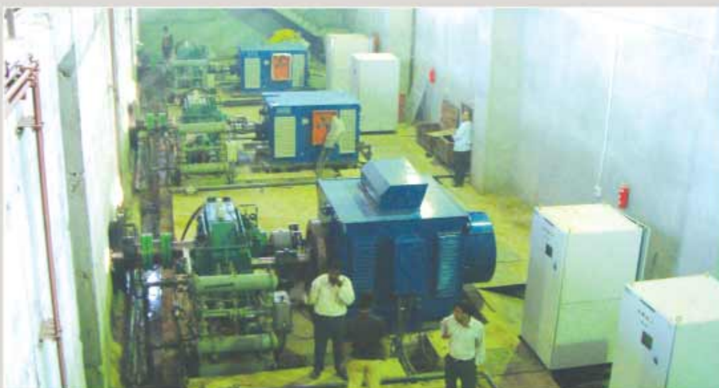
▲ A view of the TG hall
